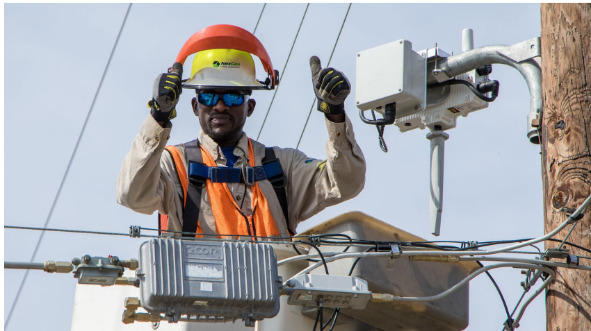
Typical Mounting of Cellular-backhaul Access Point with Battery Backup
