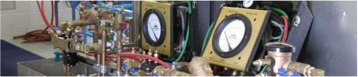
Backflow assembly testing stations in the new Backflow Testing Lab.
