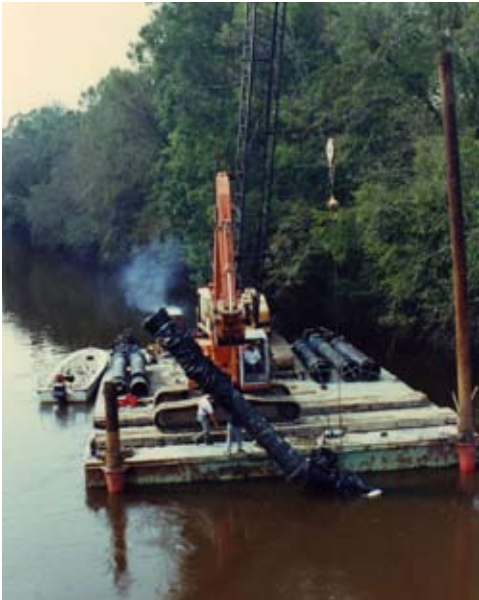
GUC's transmission main project included underwater construction on the Tar River in 1996.
