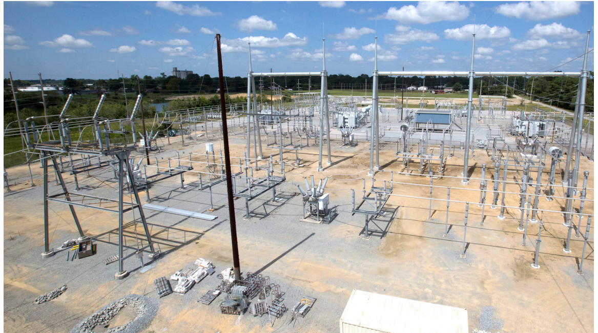
230kV Substation on Mumford Road
