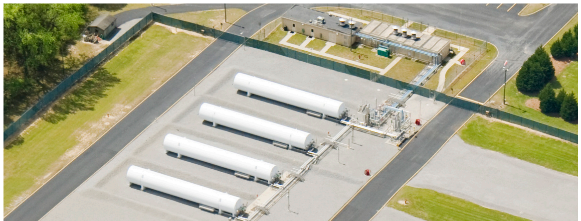
Liquefied Natural Gas Storage Facility
